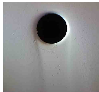
Strong sagging of paint
